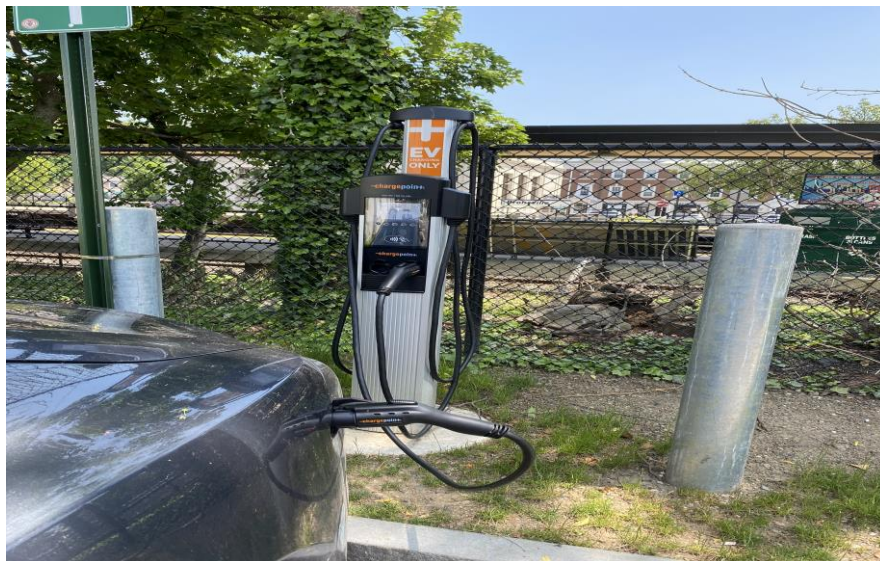
Charging station at the Parkway Road municipal parking lot
