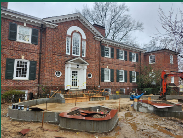
Photo of new library patio starting to take shape. Completion anticipated early this summer.
